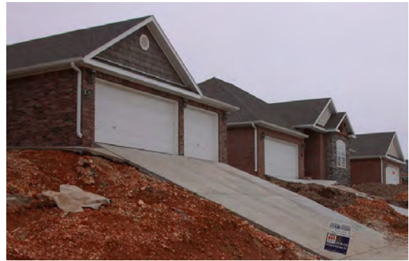
EXHIBIT 3-39 Obvious driveway grade problems
